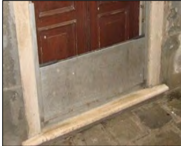
Photograph 10: Flood Barrier at Front Door of Residential Property
