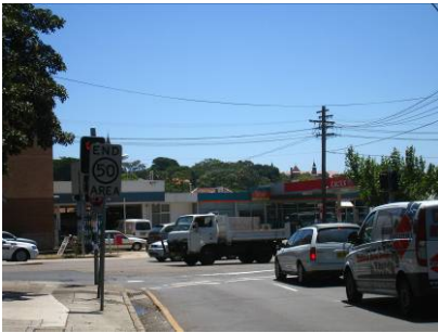
Overhead power lines at the corner of High Street and Anzac Parade
